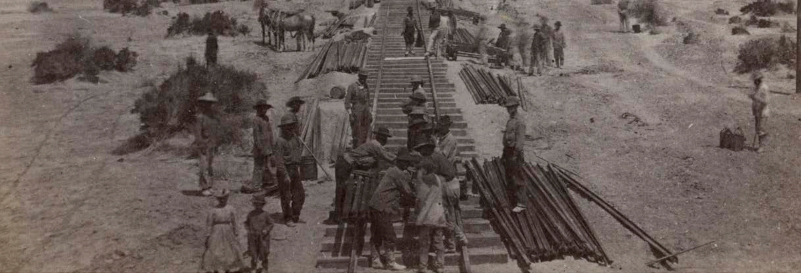
Railroad workers construct a section of the First Transcontinental Railroad on the Humboldt Plains of Nevada. (Image credit: Alfred A. Hart Photographs, 1862-1869, Department of Special Collections, Stanford University Libraries)
